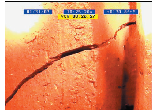
Finding cracks underground
