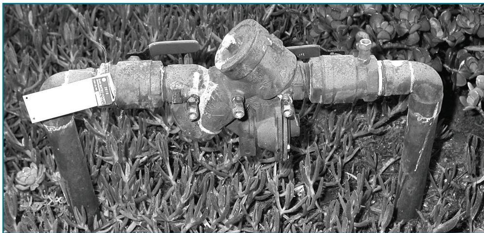
This picture shows a typical back-flow valve installation.
