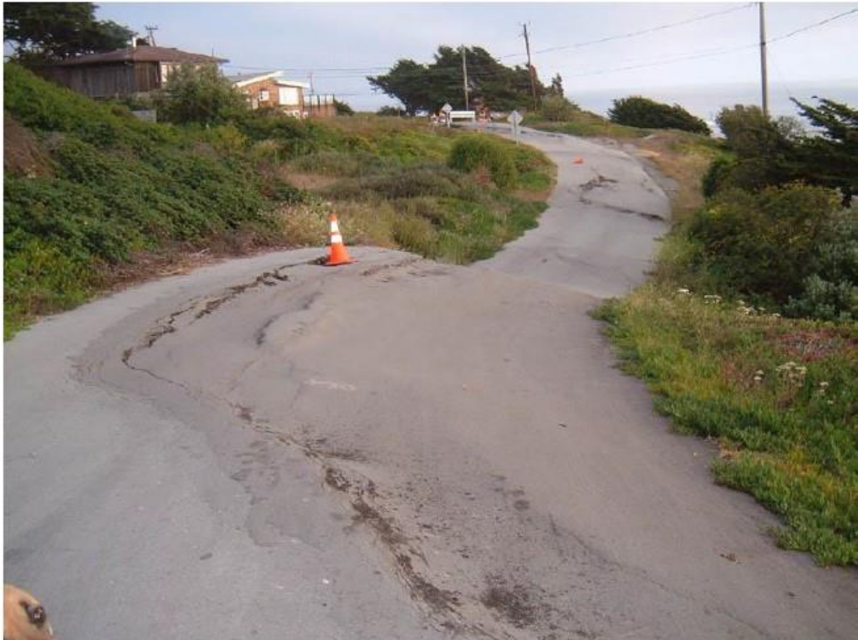
Picture 10: Slip on active scarp visible as slip line cracks in the road, as is a fault line settlement as the large dip in the road.
