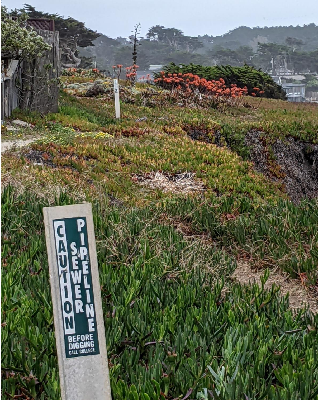
Picture 11: Slip on active scarp visible as cut in edge of cliff. Notice the sewer Caution markers. This sewer was re-aligned about 10 feet inland after this slip several years ago which caused a pipe failure.
