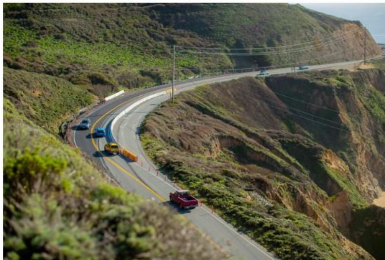
Highway 1 jogs inland near Gray Whale Cove as transportation engineers work to reinforce the roadbed and protect it from erosion. Kent Hwang / Review
