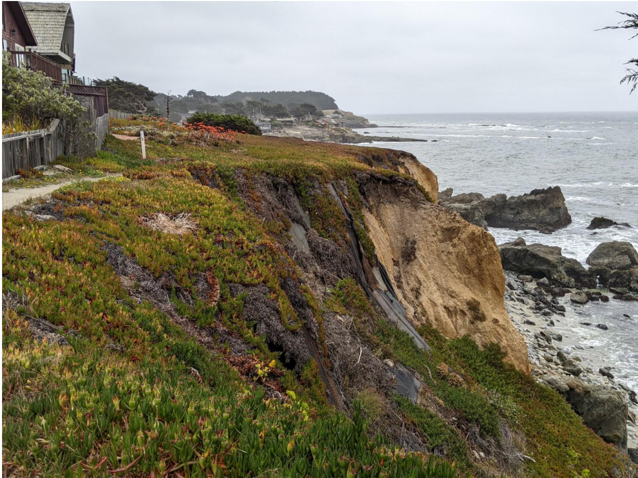
Picture 12: Larger view of the active slip of the scarp visible as curve in cliff line where soil sluffed down. Notice someone placed erosion protection fabric to try to reduce the failure rate in the soft soil area.
