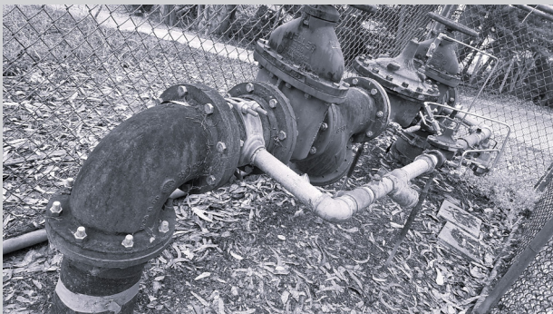
Pressure Reducing Valve Station
