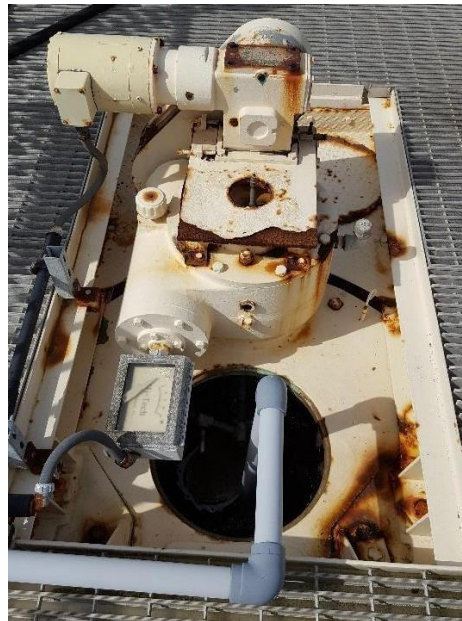
Secondary clarifier drive motor and gear reducer
