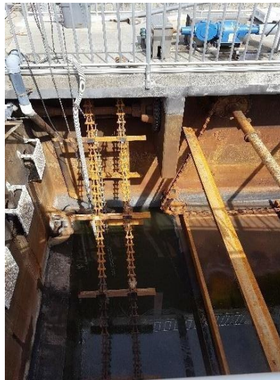
Primary clarified bottom sludge collector chain and flights
