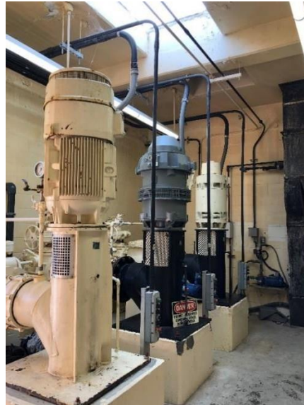
Effluent pumps 1, 2, and 3
