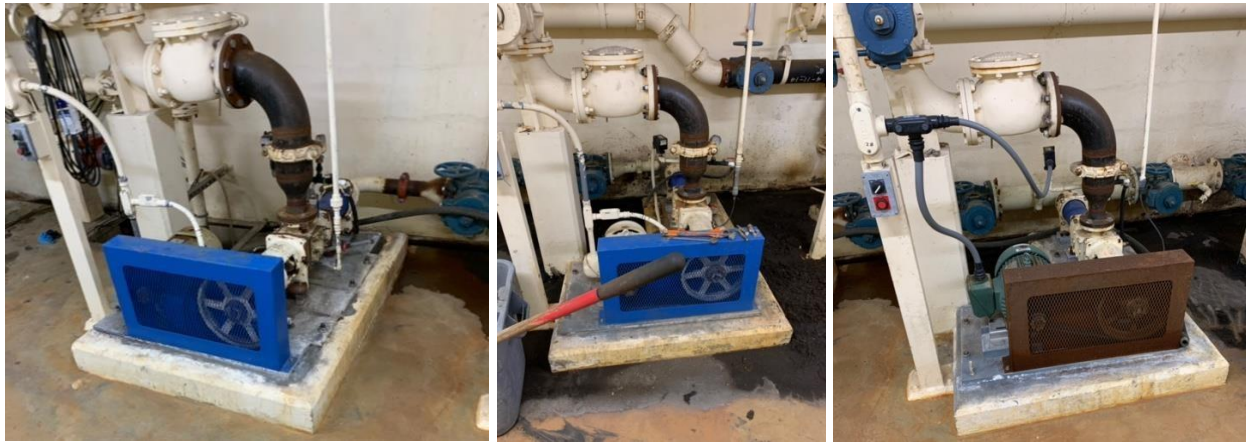
Primary Sludge Pumps 1, 2, and 3
